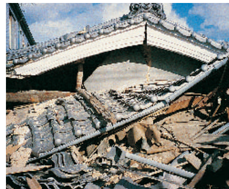
Traditional clay tile roofs are inevitably heavy weight and cause structural damage in Earthquakes
